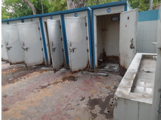
Dilapidated condition of toilets in Shakur Basti which were later cleaned and made functional due to the efforts of HLRN
