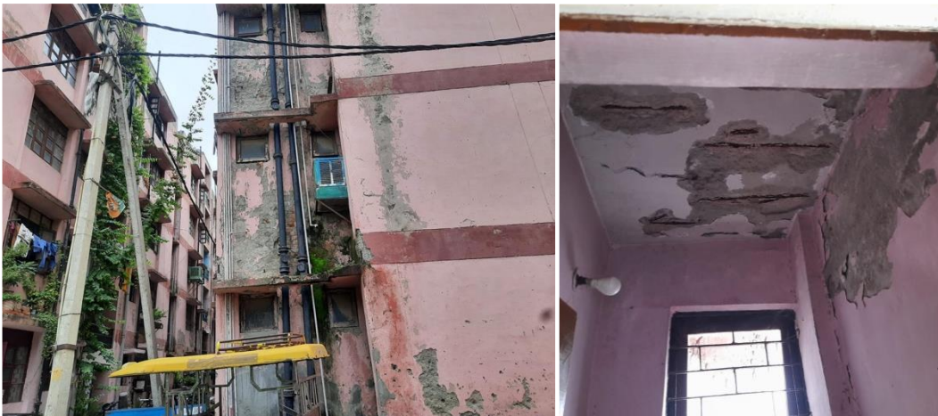
Damaged Condition of Houses at the Resettlement Site in Dwarka, Delhi
